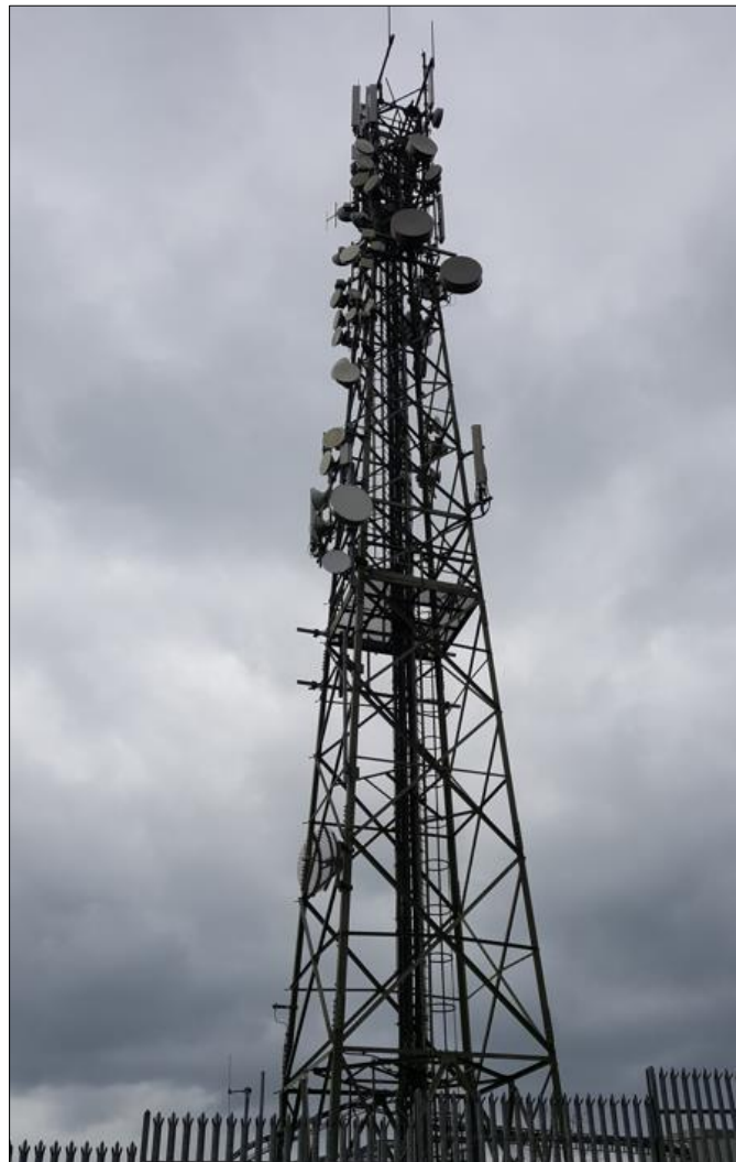
Figure 2. Telecoms Mast at Laghtseefin
