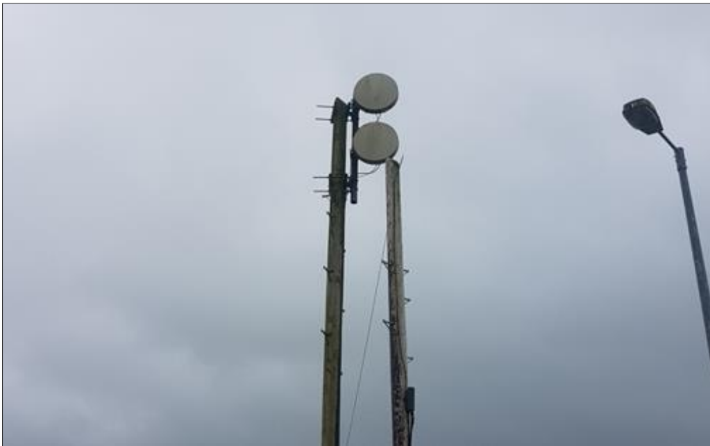
Figure 4. Telecoms Mast at Rosegreen
