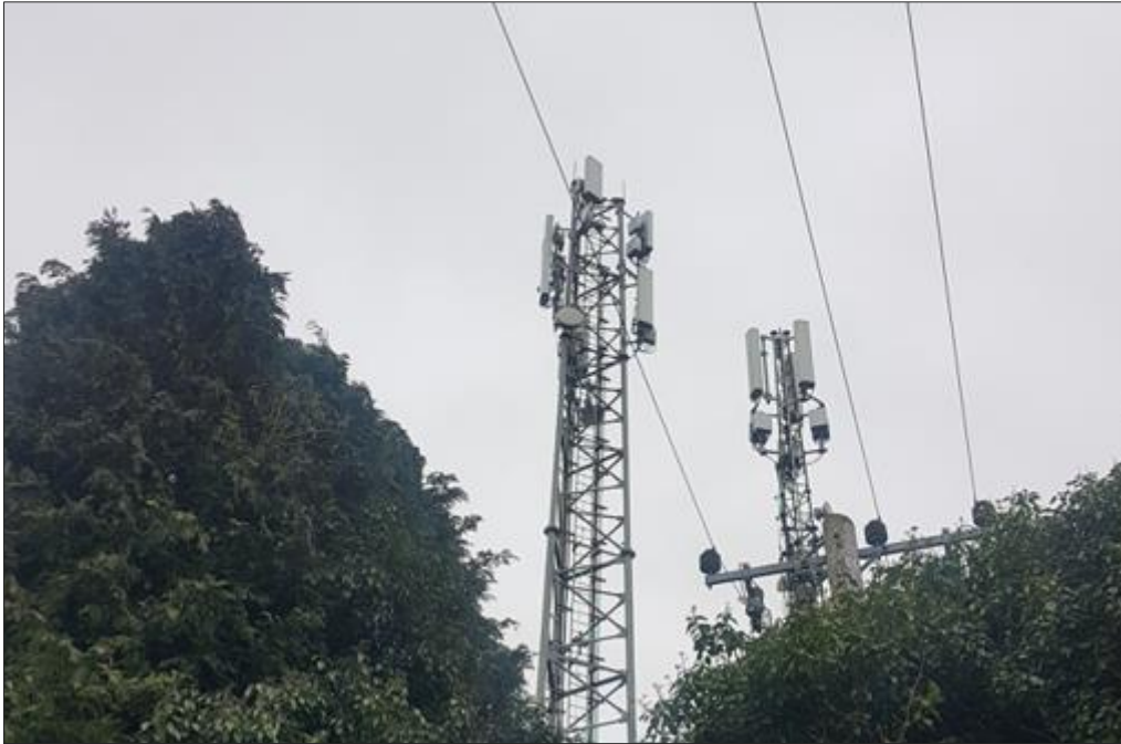
Figure 7. Telecoms Mast at Waller’s-Lot, Cashel
