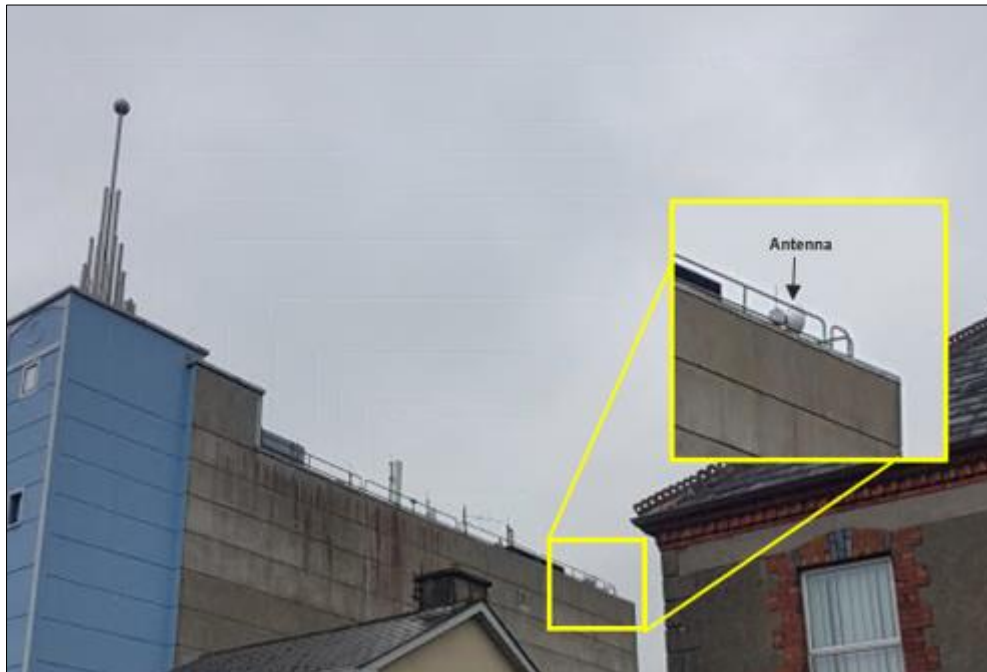
Figure 8. Telecoms Mast at Tipperary Town
