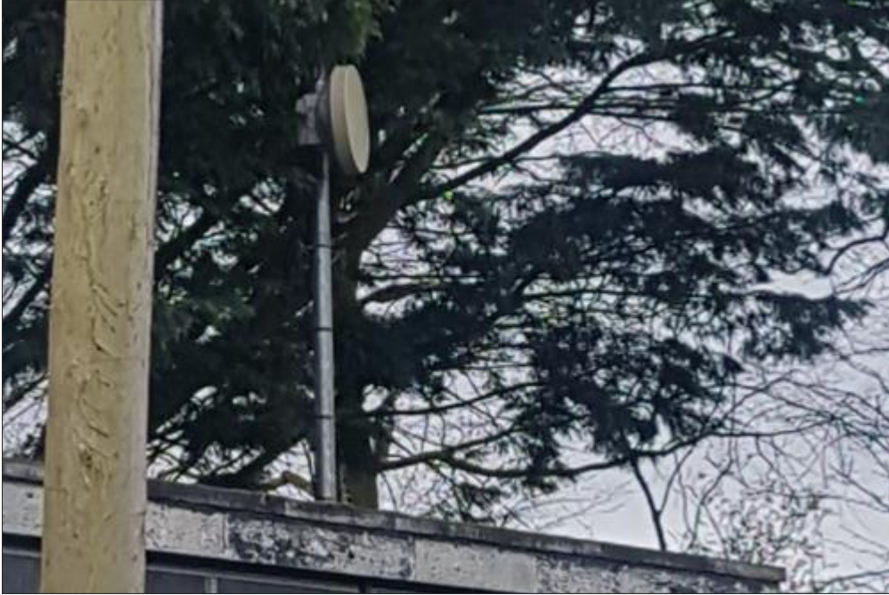
Figure 3. Telecoms Mast at Goulds Cross
